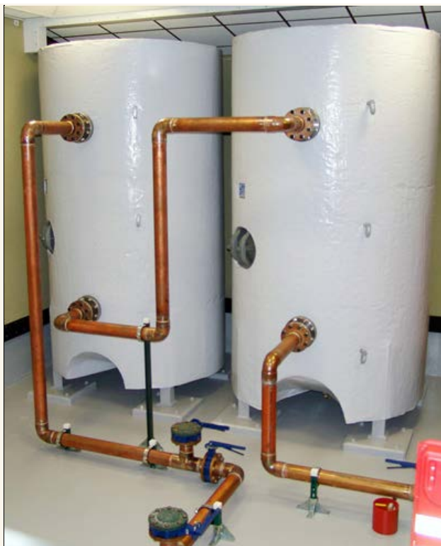
This installation photo of the chilled-water reservoir shows two 1,500-gallon storage tanks connected in series by copper pipes (before the pipes were insulated to prevent condensation in the computer room). Chilled water from the tanks is used to prevent bluefire from overheating in the event of a power outage that could momentarily disrupt the supply of chilled water.
