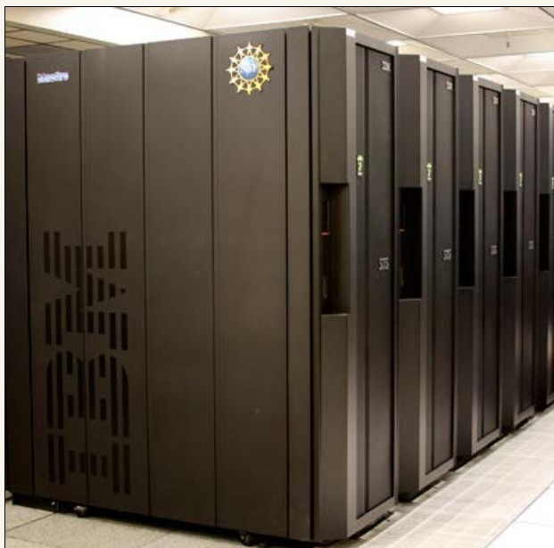
During FY2008 NCAR took delivery of the first IBM Power 575 Hydro-Cluster supercomputer ever installed, continuing a 30-year tradition of providing a sustainable high performance computing environment to the atmospheric sciences community. The bluefire system is based on the world's fastest microprocessor, the IBM POWER6 dual-core chip with a 4.7 GHz clock speed. In June 2008 bluefire was ranked as the 30th most powerful computer in the world by the Top500 project.
