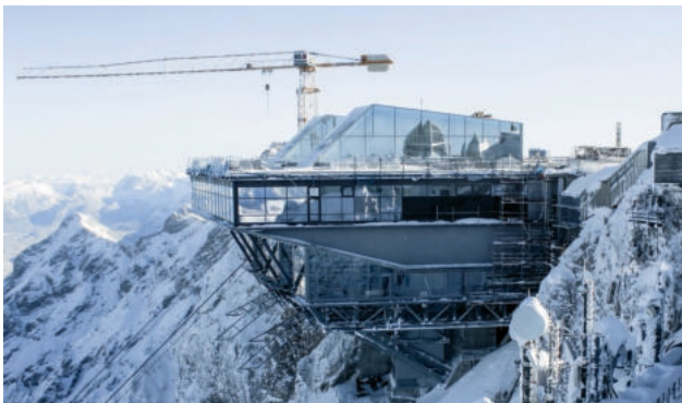
Fig. 19: Construction site of the new summit station for BZB’s “Seilbahn Zugspitze” (“Cable Car Zugspitze”)
