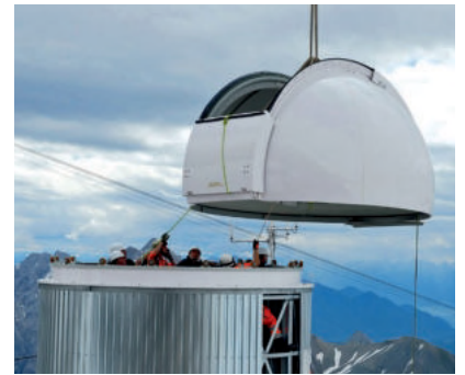
Fig. 26: Installation of the large laser tower for the RAMAN-LIDAR on the roof platform of the UFS building (2010)
