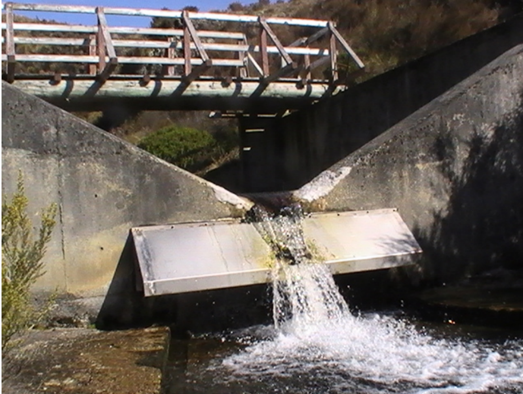
Fig. 4.5 The stainless steel migration barrier installed by the DOC in 2008 (photo: Josh Tabak)
