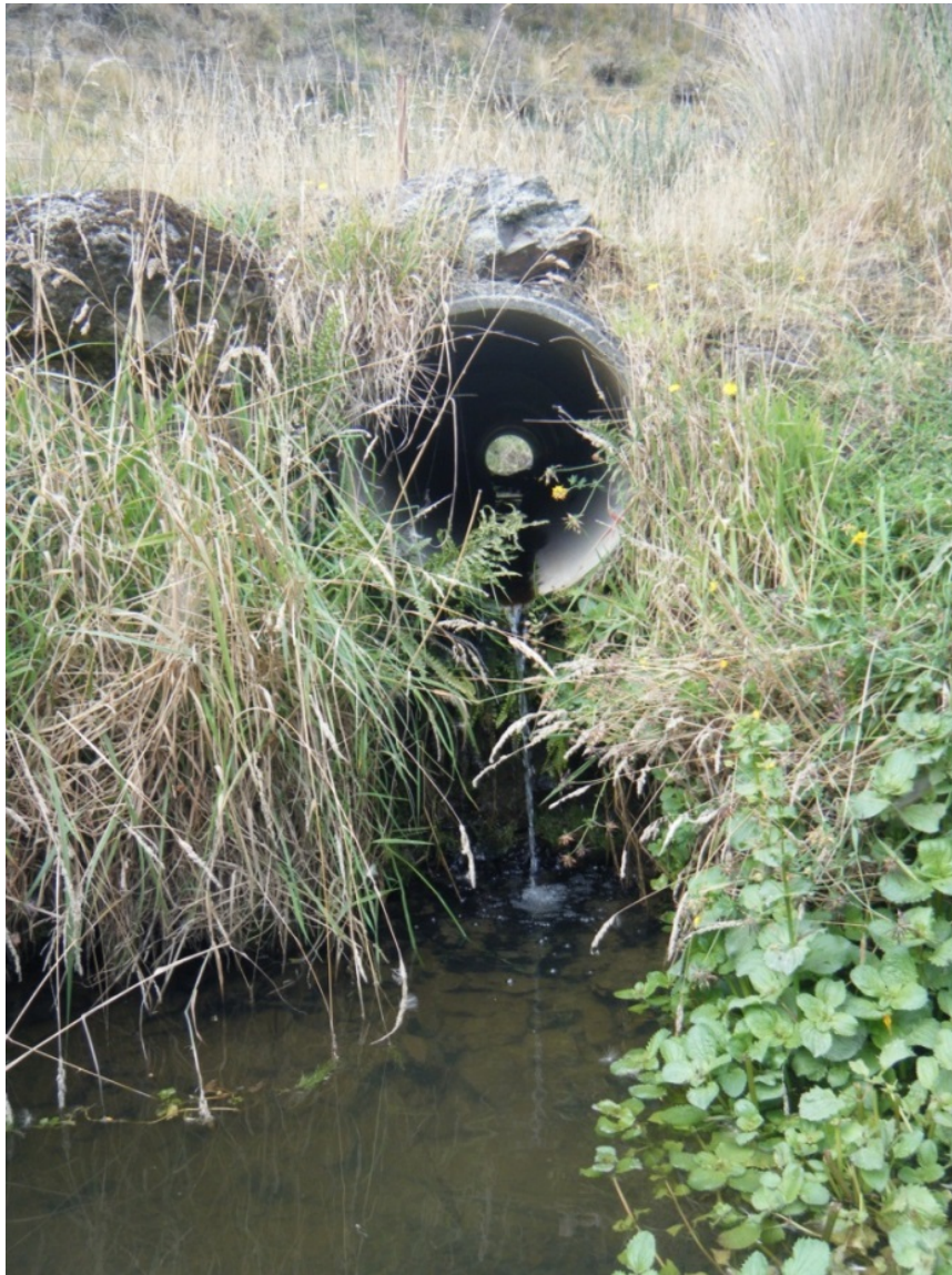
Fig. 2.1 A perched pipe culvert, Tokomairiro River tributary, Dunedin (photo: Josh Tabak)
