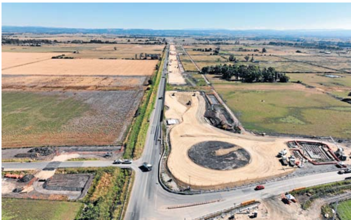
A roundabout at the intersection of Ballarto Road and Healesville-Kooweerup Road is underway.
