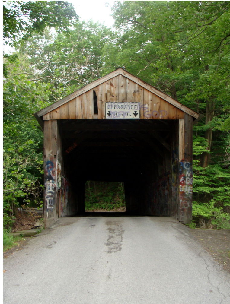
Yet another photo showing the extent of vandalism -- July 2008
