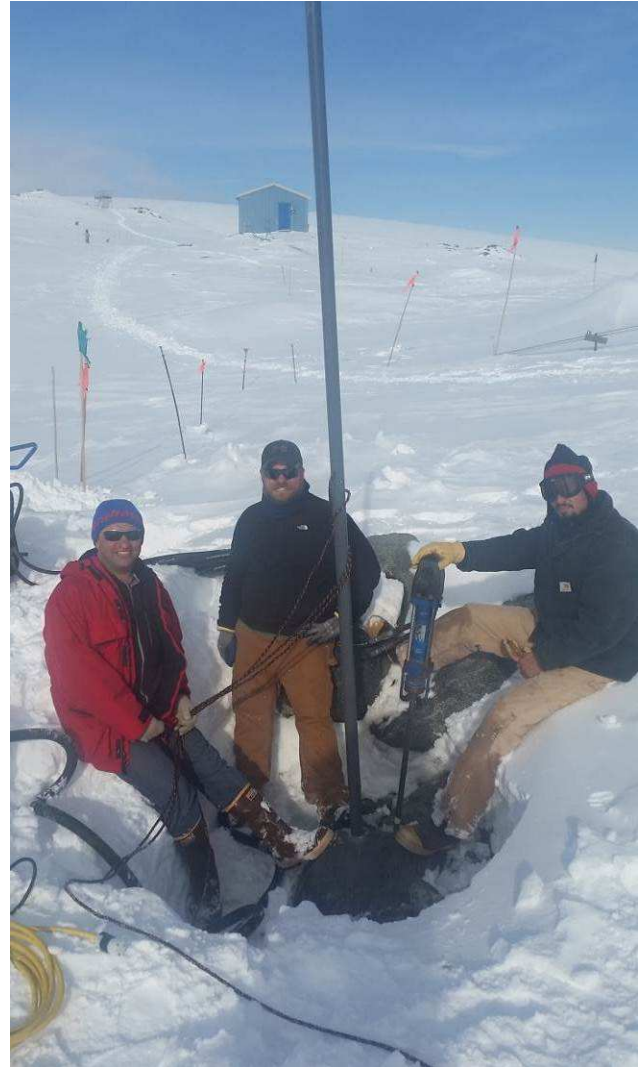
Figure 3. Anchor installation crew led by Joe Bissonnette (right) and Jeff Keller (center). Guy bolts and antenna masts were mounted in rock with help from the big drill. P.I. Vadym Paznukhov (left) looks on.
