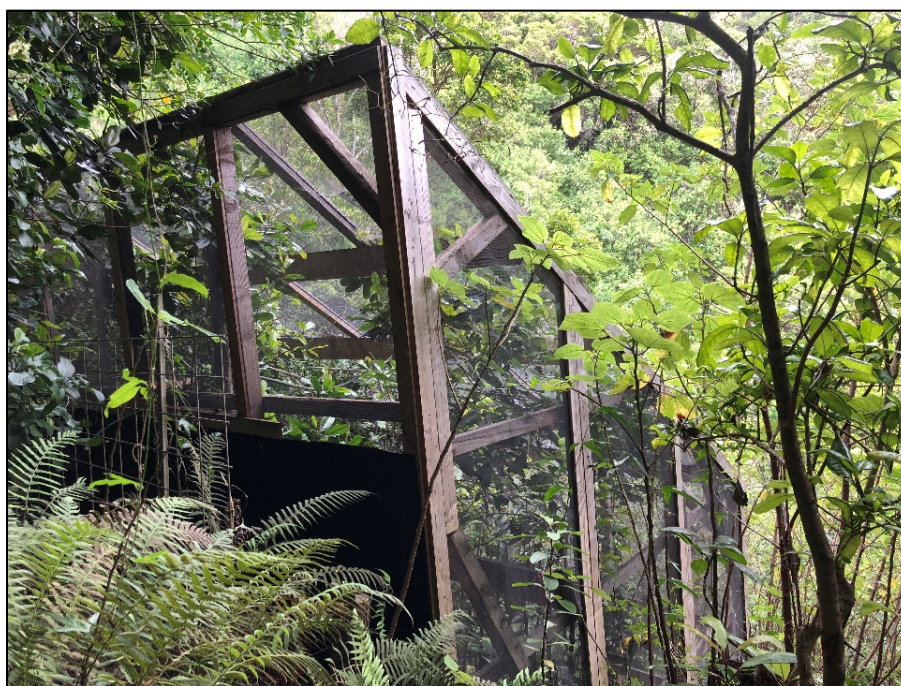
Figure 4. Photograph of the temporary enclosure structure at Ekahanui, July 2018
