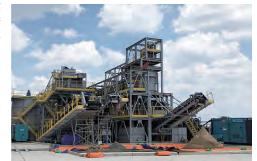
Soil washing plant to remove dioxins at Bien Hoa Airport in Vietnam
