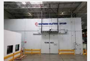
Dedicated Pharmaceuticals Temperature-Controlling Cabinet (Chicago)
