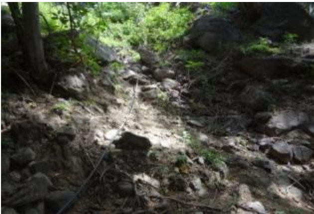
El Gavilan, construction of the structure for retention or harvest of rainwater and water flow
