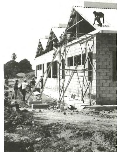
Factory shells under construction in Dominica are tangible testimony that the CBI's incentives are at work.
