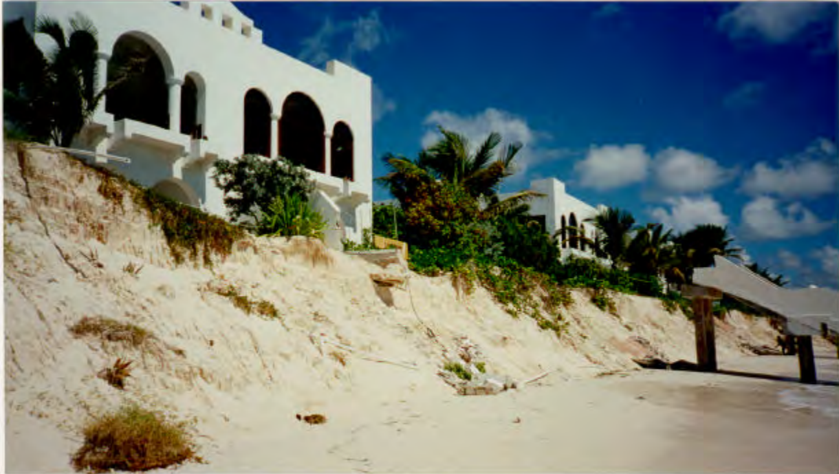
Photograph 10. Eroded dunes at Maunday's Bay, Anguilla, October, 1997. Note the concrete steps are detached from the villas, and the villas are perched on the edge of an unstable 'cliff' of sand.
