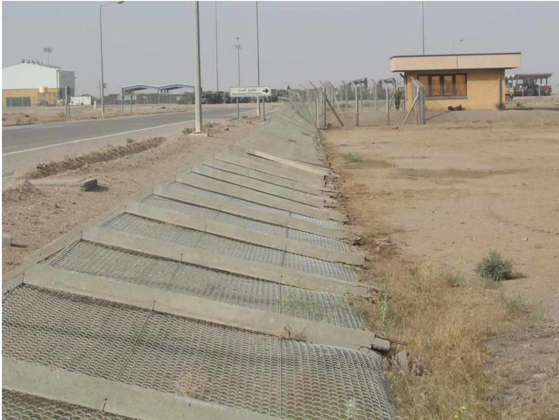
Security fence posts damaged by salt attack
