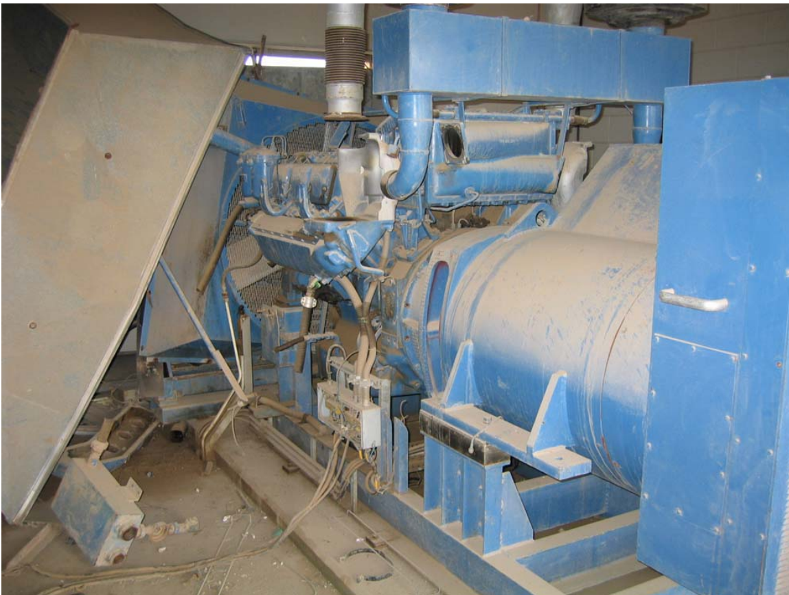
Damaged generator set at Field Electrical Centre
