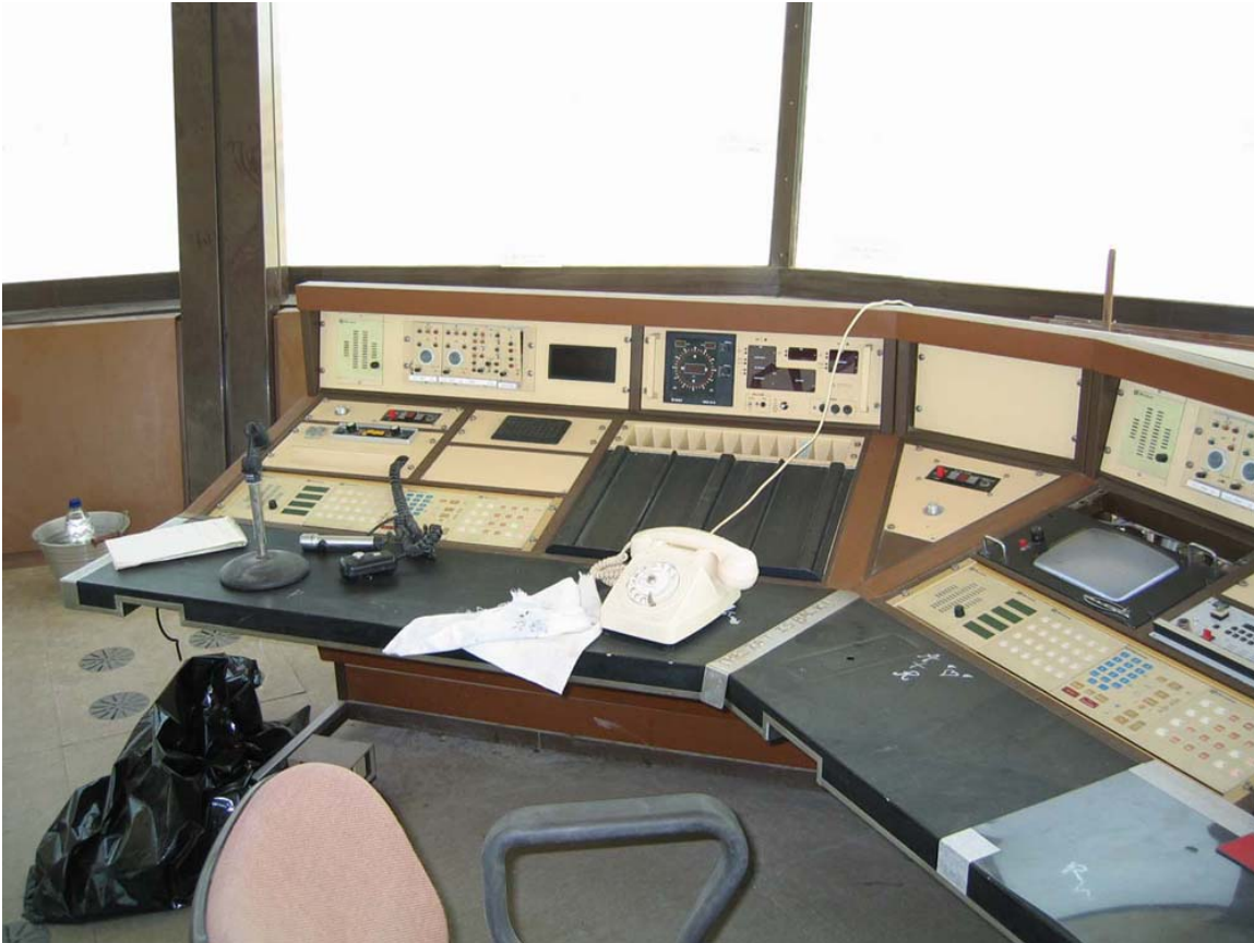
Control tower - consoles
