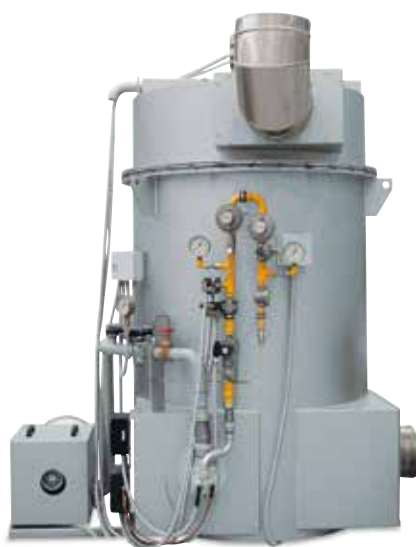
Thermal afterburning system
