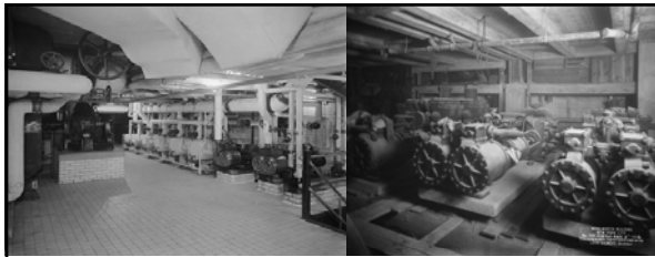
"...A powerful fire-pump forms part of the Building's thoroughly complete fire-fighting equipment. This pump, located in the sub-basement, is capable of delivering 500 gallons of water per minute at the fifty-eighth story against a head pressure of 820 feet, and on account of the protection thus afforded neighboring properties, the owners have, in some cases, been able to secure substantial reductions in their fire insurance premiums..." RE: excerpt from "The Cathedral of Commerce" Left: caption: "Woolworth Building, pump room" Right: caption: "Woolworth Building, engine/pump room from west end" 363
