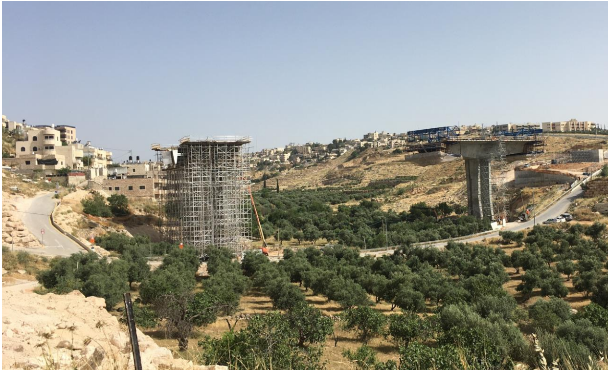
The construction of a bridge at the Eastern Ring Road, Sur Baher, East Jerusalem, May 2020
