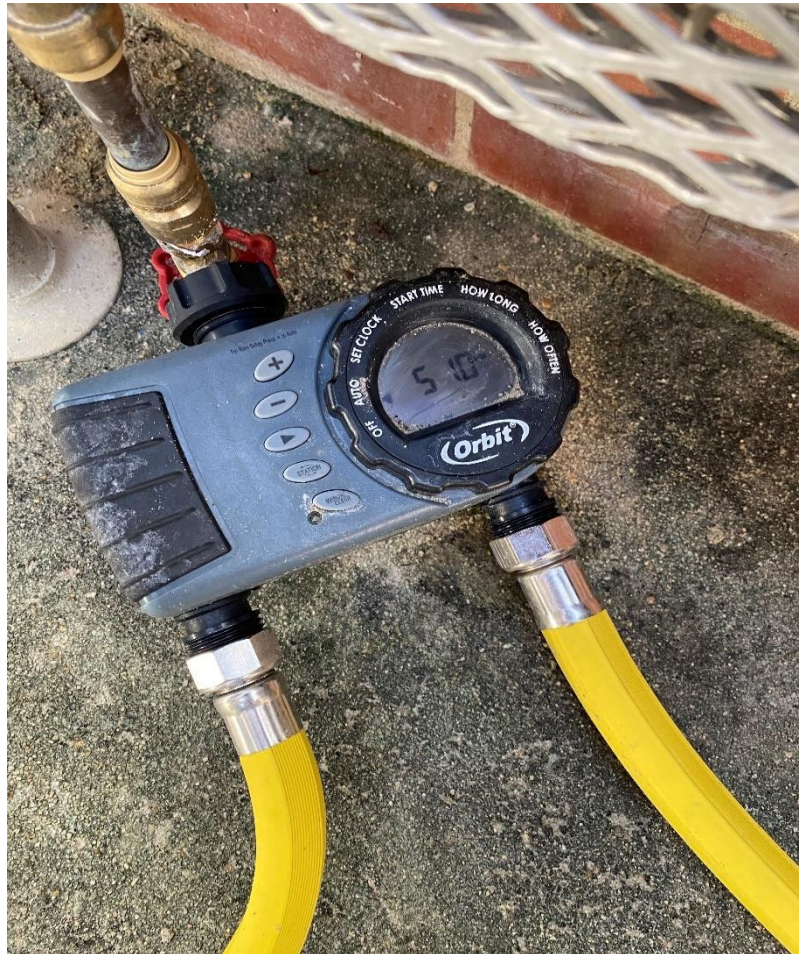
One control box for two benches.
