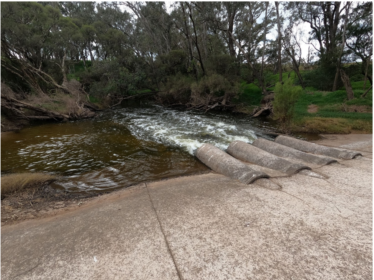
Figure 5 Pipe culvert road crossing ~1km downstream of Murray River Farm downstream site.
