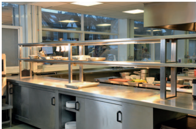
Figure 3.2 Example of a hotplate area
