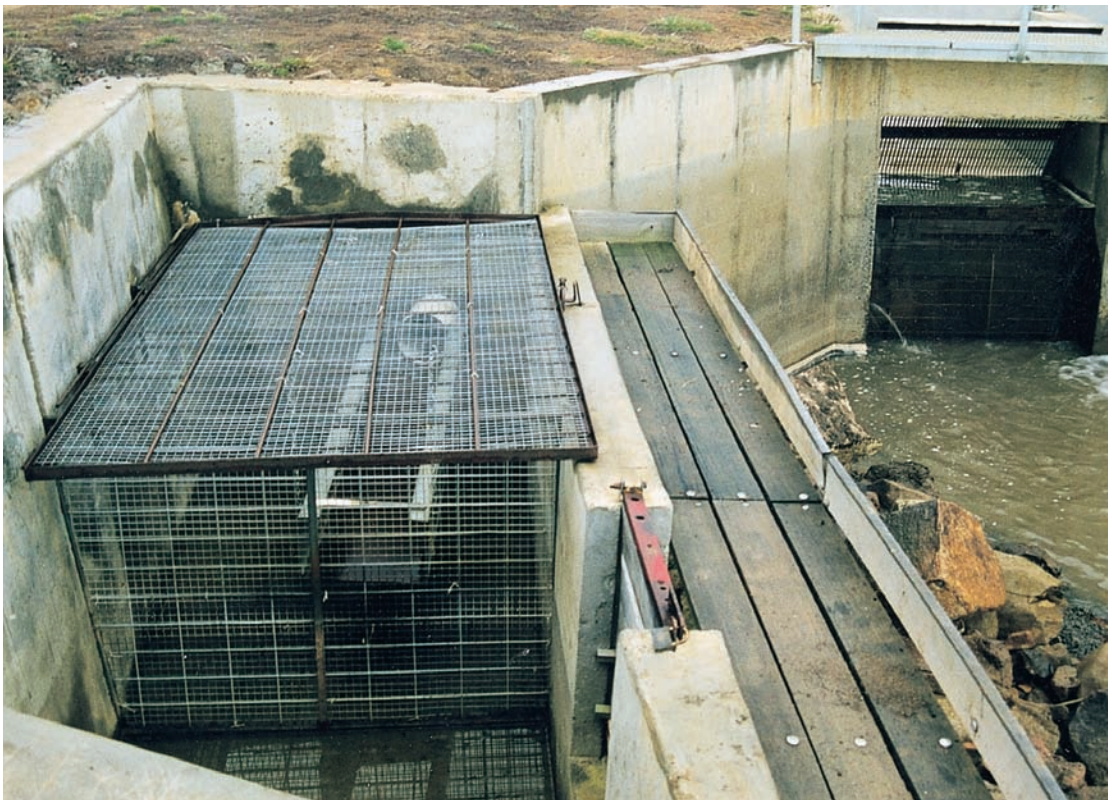
Outlet weir from Lake Sorrell showing flow-through screens and trap which have been constructed to restrict carp movement. Source: A. Brumley, East Gippsland Institute of TAFE.
