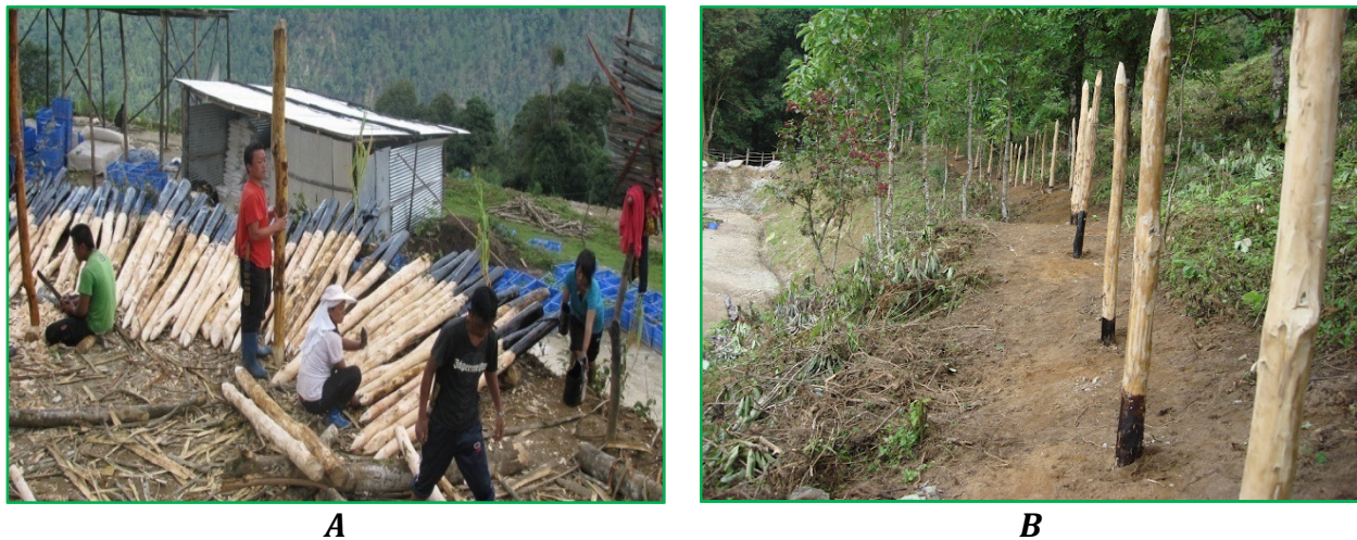
Figure 8: Bark removing and painting of wooden poles (A); Wooden poles fixed in the soil (B).
