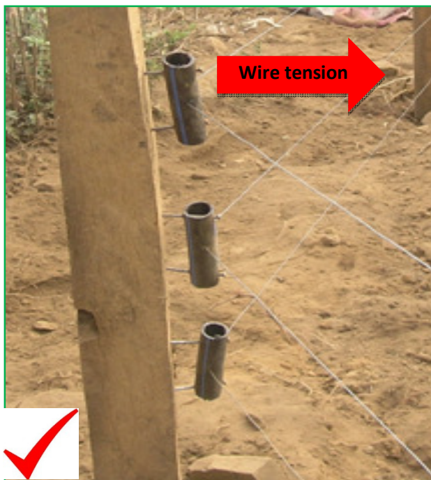
Figure 14A. HDPE insulator fixed in opposite direction of the wire tension
