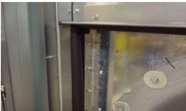
Figure 13. Duct strip cover
