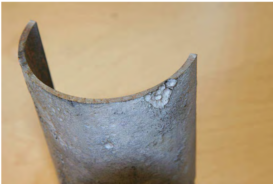
Figure A-2 Shell segment of forged mercury container cut through area with maximum metal loss
