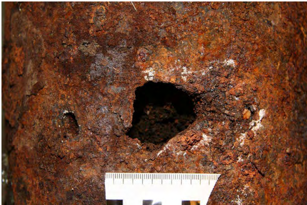
Figure A-8 Close up of pressurised gas cylinder wall penetrated by corrosion
