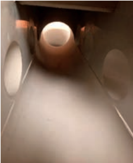
Smooth bore internal branch inlets
