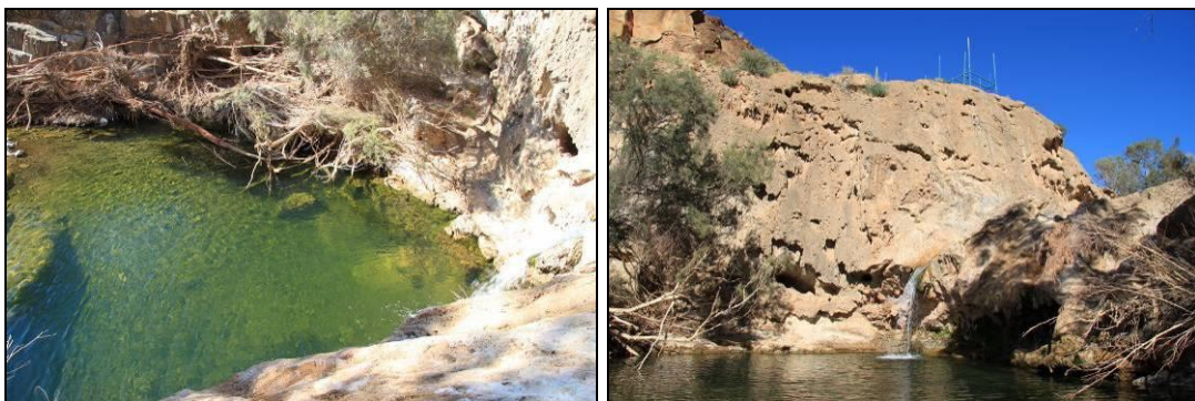
Figure 17. One of the deep pools at Moro Gorge with the viewing platform still being constructed (right).
