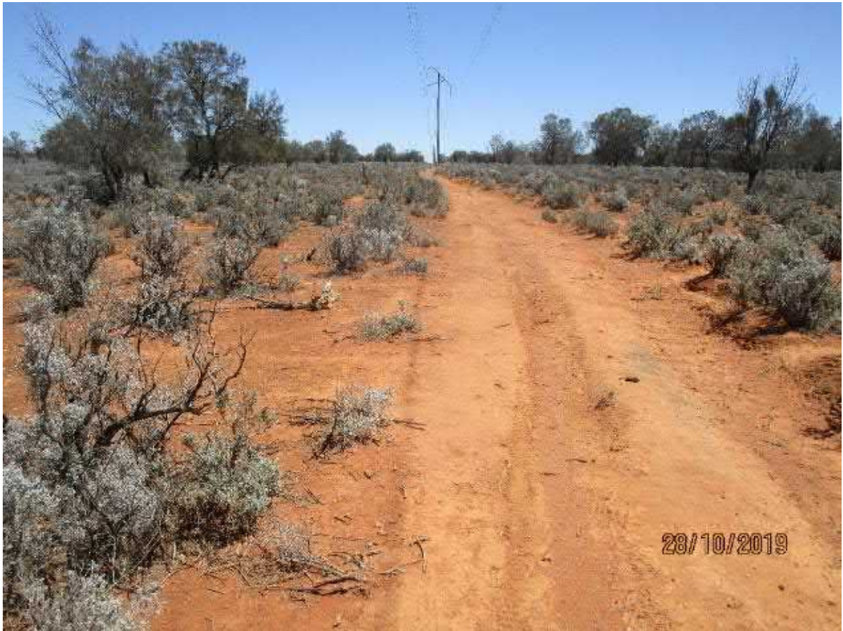
Plate 3-35: Site 5c, three metre clearance for existing track plus additional past clearance of Casuarina pauper (Black Oak) up to 10m either side of track (facing west)
