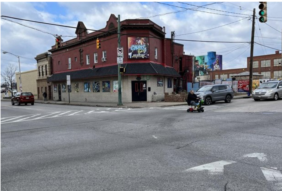
Intersection of E. Lombard and Haven Streets showing faded crosswalk markings and an individual using mobility scooter crossing the street. (January 18, 2022)
