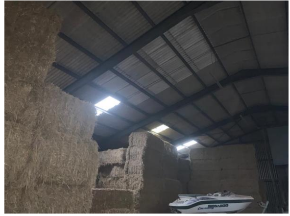
Photo 2: Internal view of building, with steel girders supporting corrugated cement fibre board
