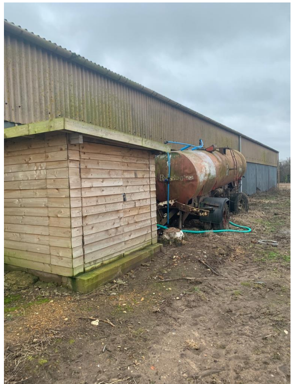
Photo 4: Small, modern, single skinned shed and stored farm machinery along part of western façade
