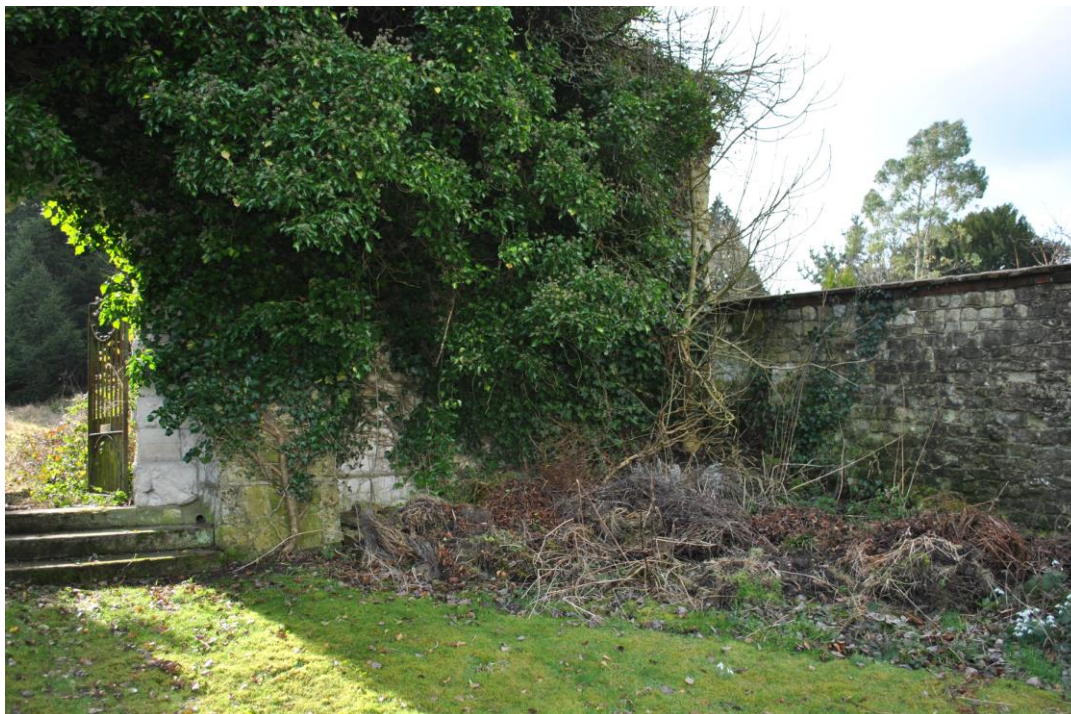
West end of the curtilage wall meeting boundary wall to Bordean House. The growing ivy is taking hold of the wall causing severe deterioration of the malmstone.
