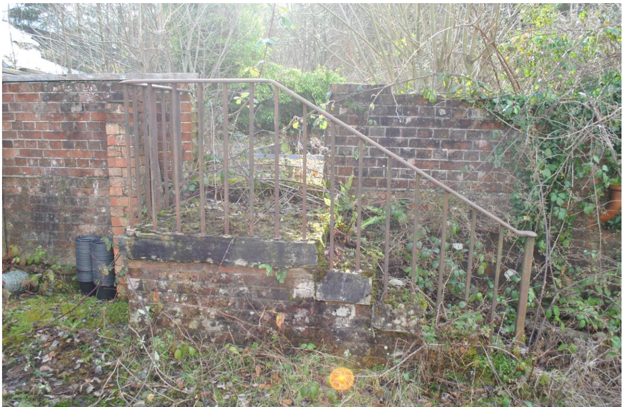
The base plinth walls and entrance steps are all that remain of the western greenhouse.
