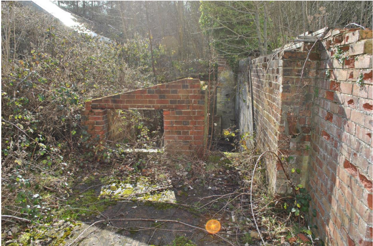
The remains of the boiler room and chimney between the two greenhouses. Presumably used to provide heating for the greenhouses.
