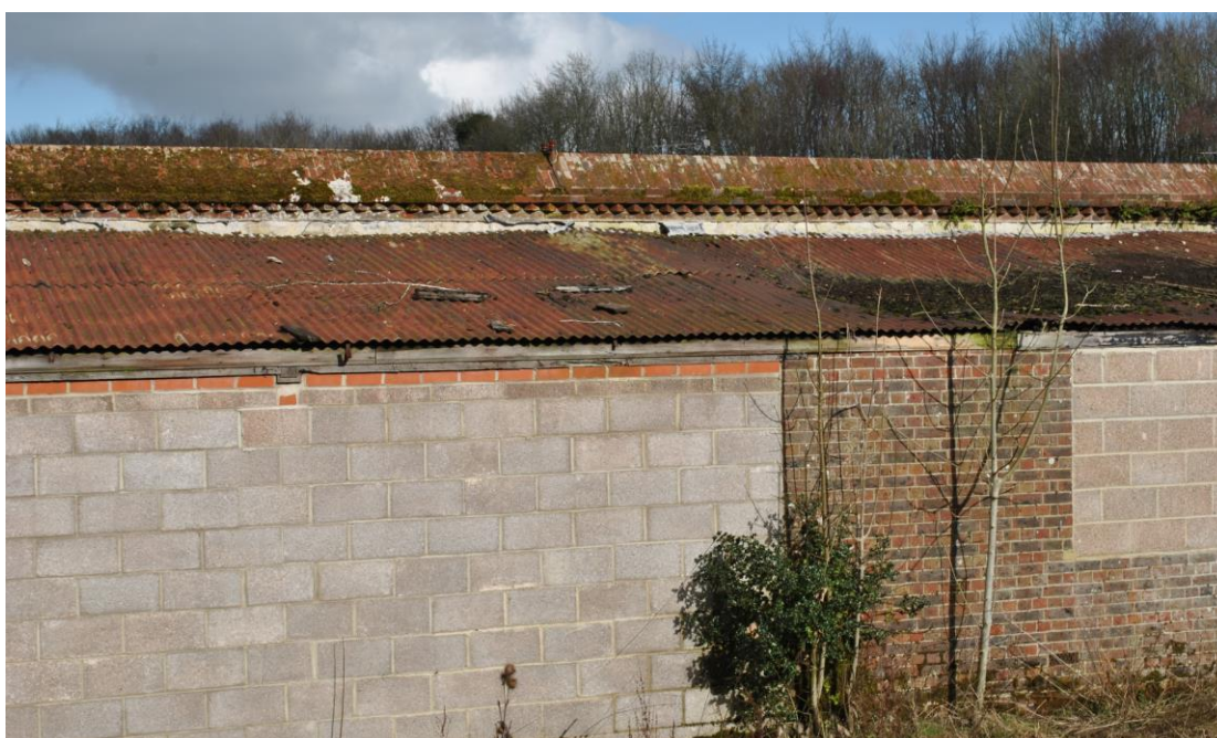
The south side of the Wall has an attached outbuilding of brickwork/blockwork walls and corrugated metal roof sheeting.
