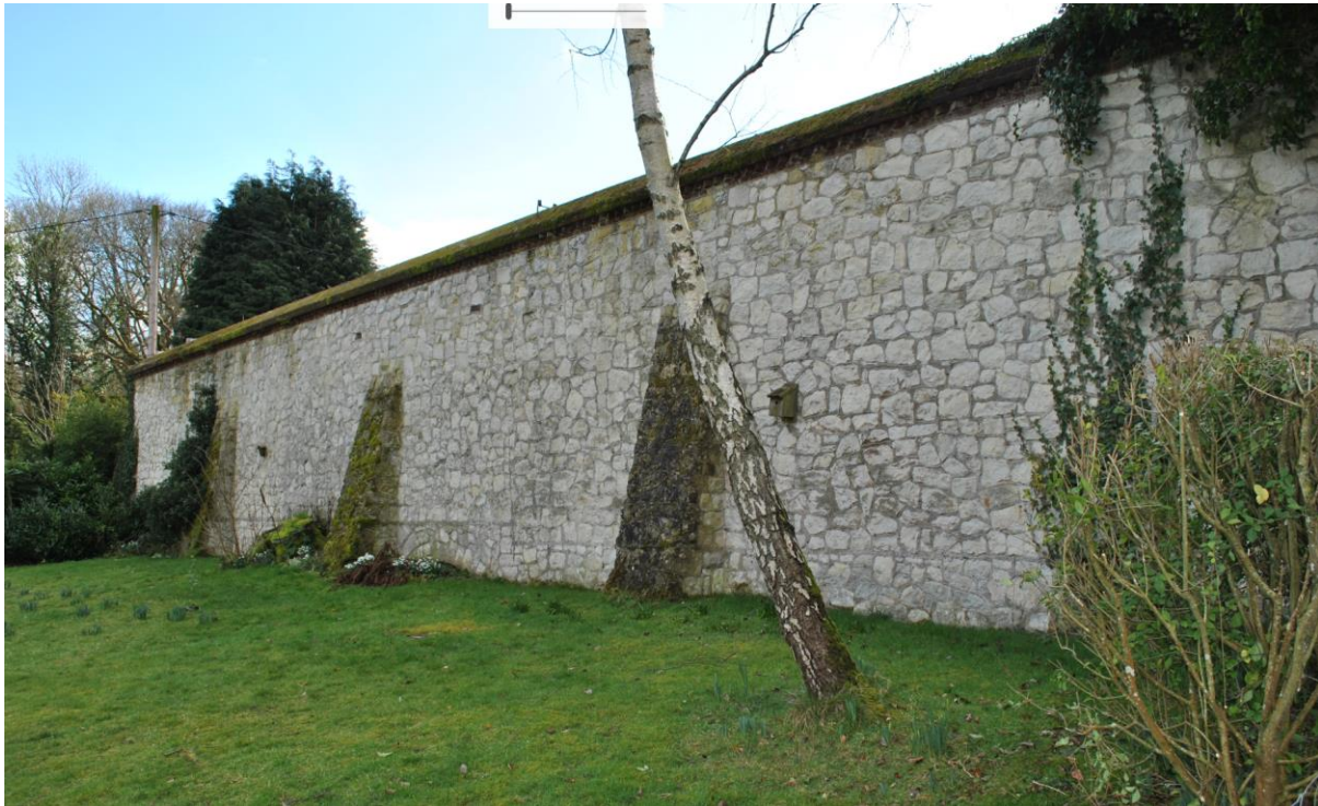
The main Malmstone curtilage wall with brick dentil detail just below the pitched brick capping to the top of the wall.
