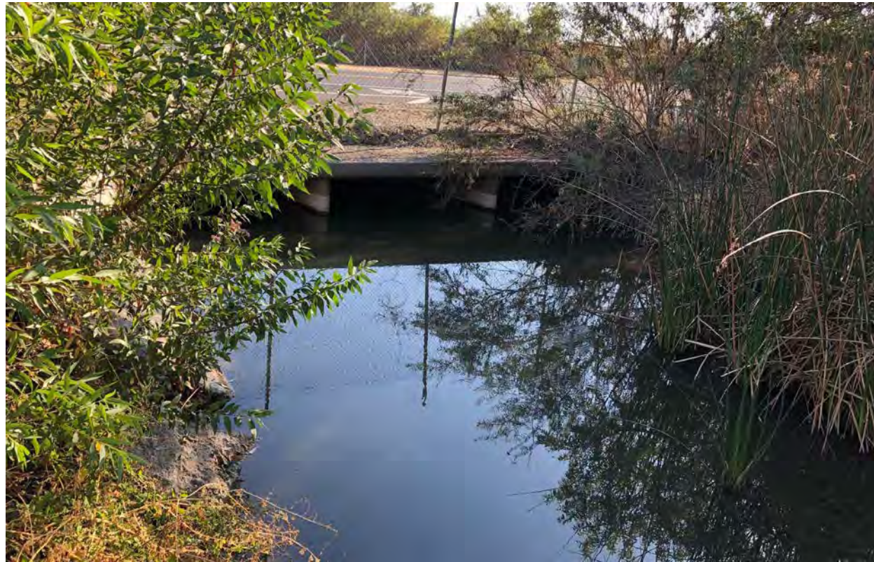
Photograph 1: Culvert at Campus Drive where water is discharge to SJMR from Irvine Ranch Water District.
