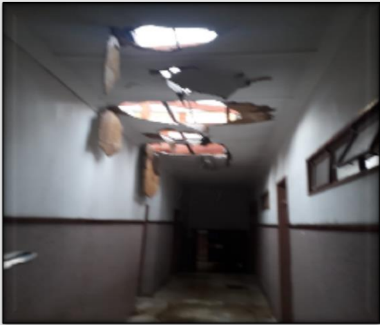
Damaged ceiling due to blown off roof during rain storm
