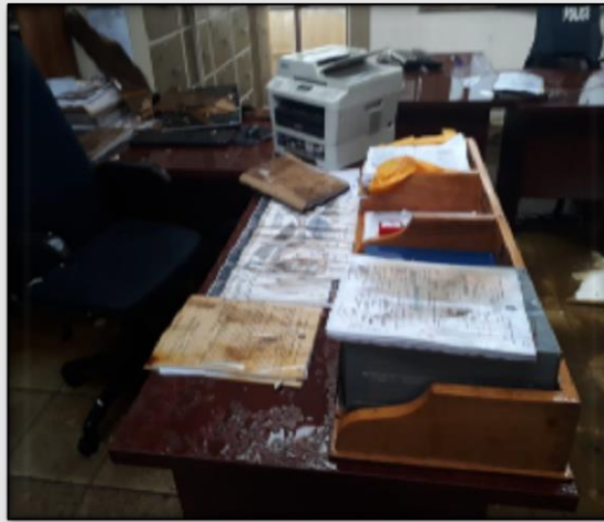
Flooded offices and damaged state items
