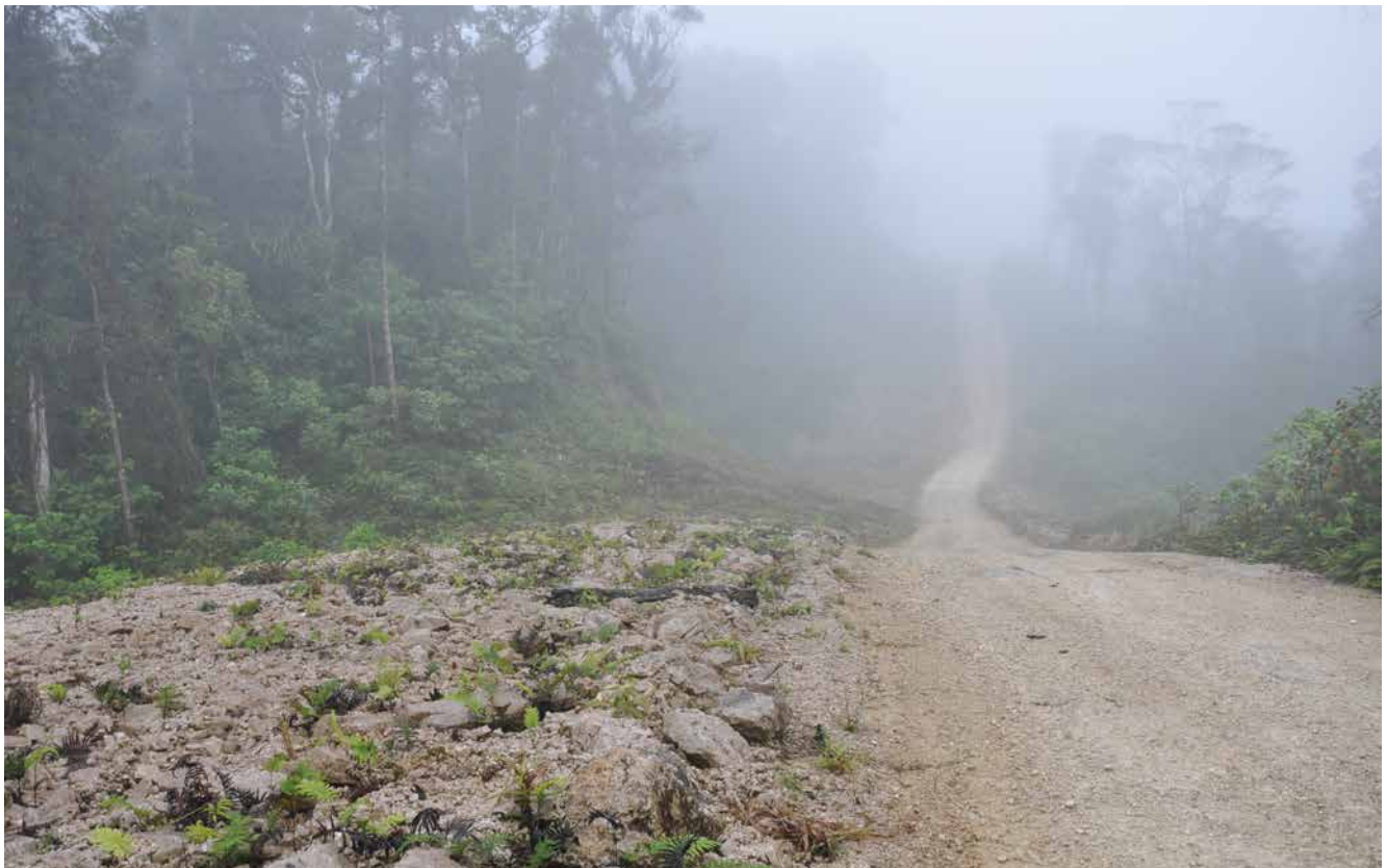
Figure 8. Linear infrastructure at KP107 in BAA 2. Note the sharp boundary between the ROW clearing and adjacent forest on the left.
