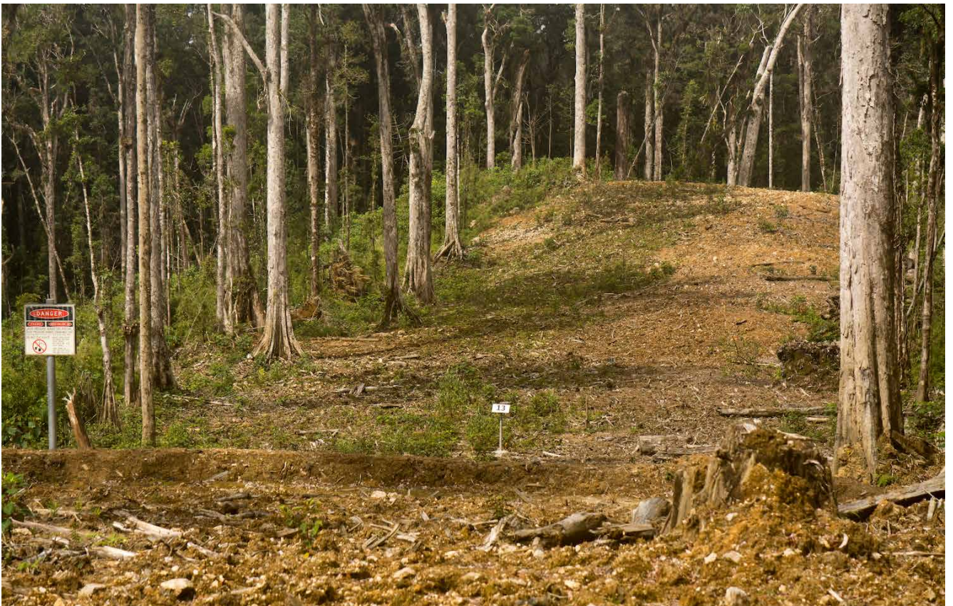
Figure 1.4. The pipeline ROW in BAA 1. The plot PLANT D is situated in the background.
