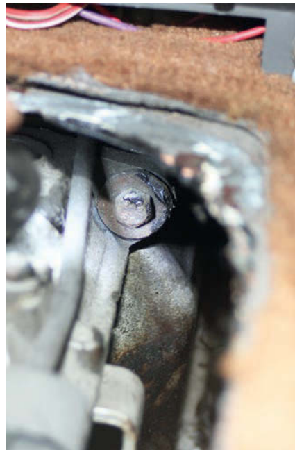
10 Now we could shine a torch in and see where the unwanted movement was coming from. This is one of two bolts that go forwards through the remote housing and into the gearbox itself.
