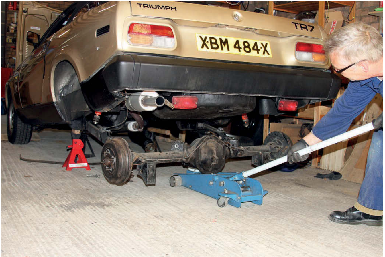
9 Ready to pull out the axle – note that the hard brake lines have already been replaced with copper pipe, one running from the flexihose to the offside brake and another running from that across to the nearside brake.
