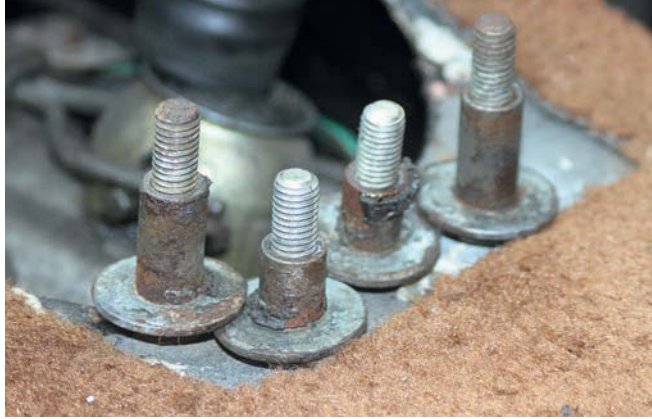
12 Taking the fixing bolts out showed that they went through metal bushes, and had large flat washers that stopped the housing from actually slipping off over the bolt heads.
