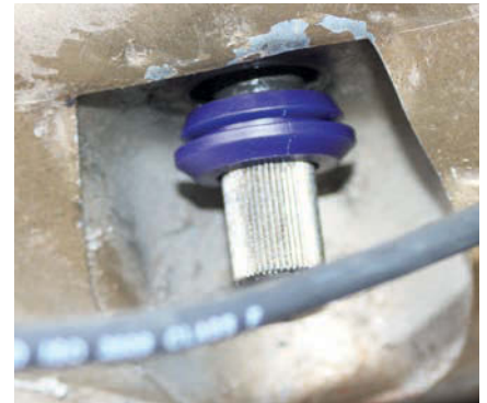
7 Unfortunately, there was no way that the bush could be pushed up the shaft and squeezed through the hole in the bulkhead.
