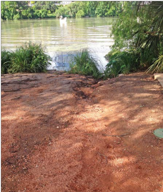
Figure 3.7: Runoff from infrastructure is causing rill erosion and erosion of trail material at Auditorium Shores.
