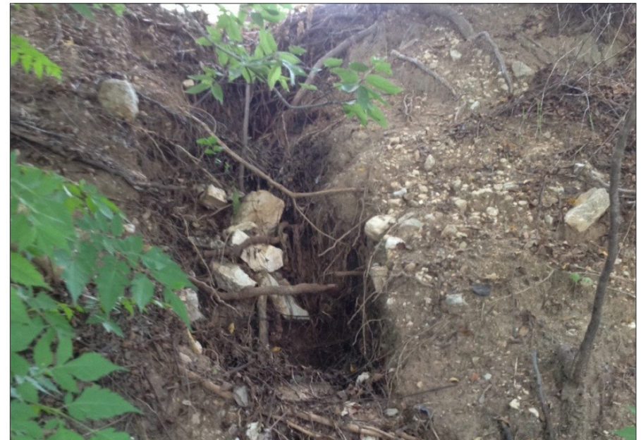
Figure 4.19 (Below): Gully erosion west of Congress Avenue Bridge.
