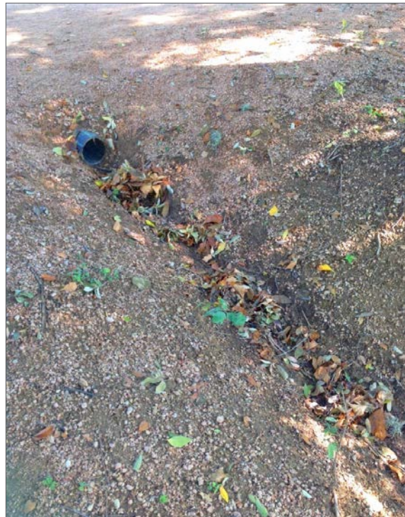
Figure 2.52: Rill erosion often occurs where culverts carry water under the Trail without armoring below.
