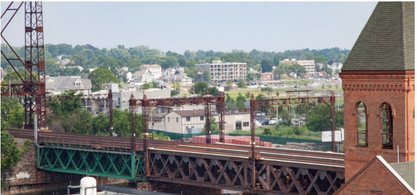
Figure ES-4: Walk Bridge in Norwalk, CT. Plans include replacing the bridge to improve speeds and reliability.
