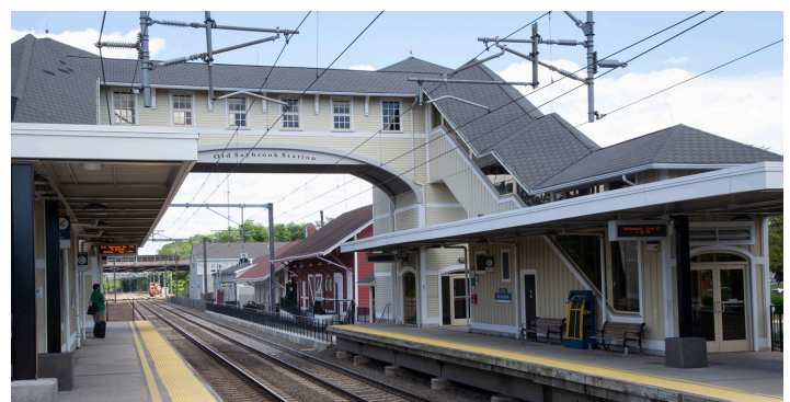
Figure ES-8: Railroad electrification infrastructure at Old Saybrook Station
