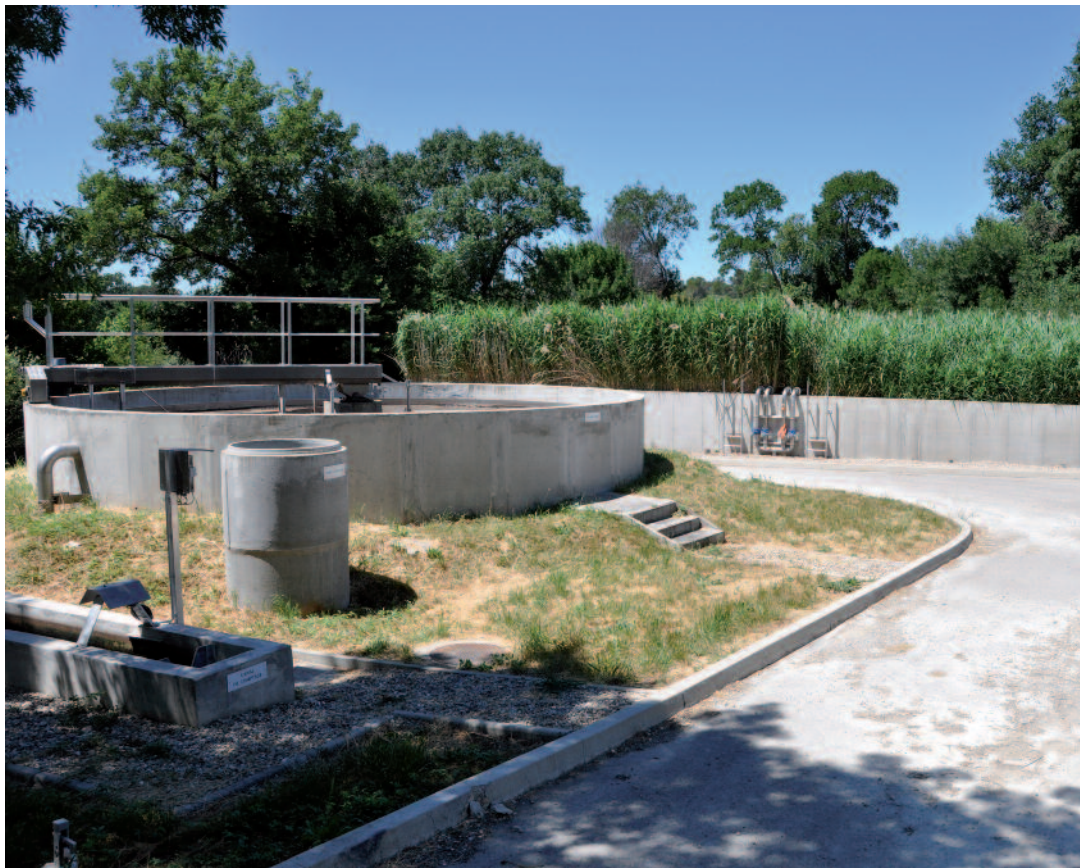
Figure 3. Water treatment plant using Phragmites australis in southern France. Photo © Brigitte Poulin, Tour du Valat.
