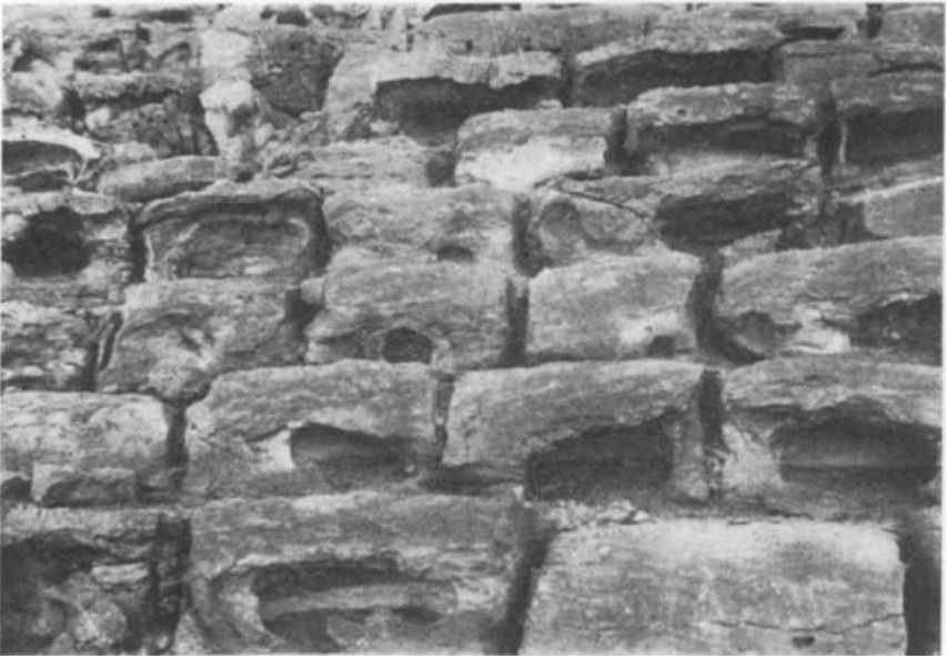
FIG. 6. — Wind erosion of limestone blocks at the upstream side.
