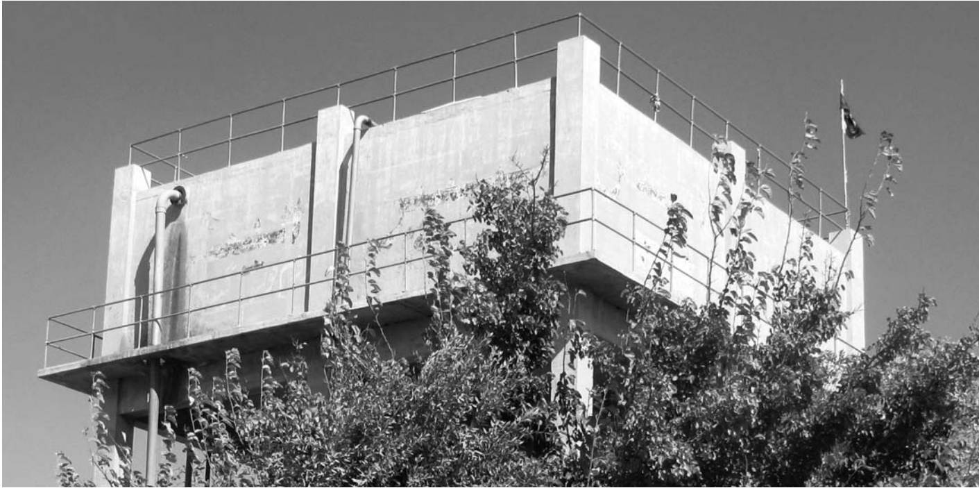
PHE water supply tank, Pishin
