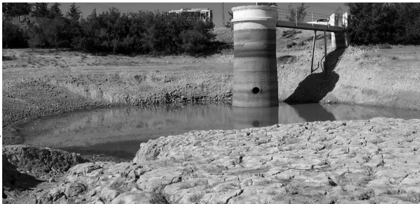
Bund Khushdil Khan, a drought-dried water storage dam
