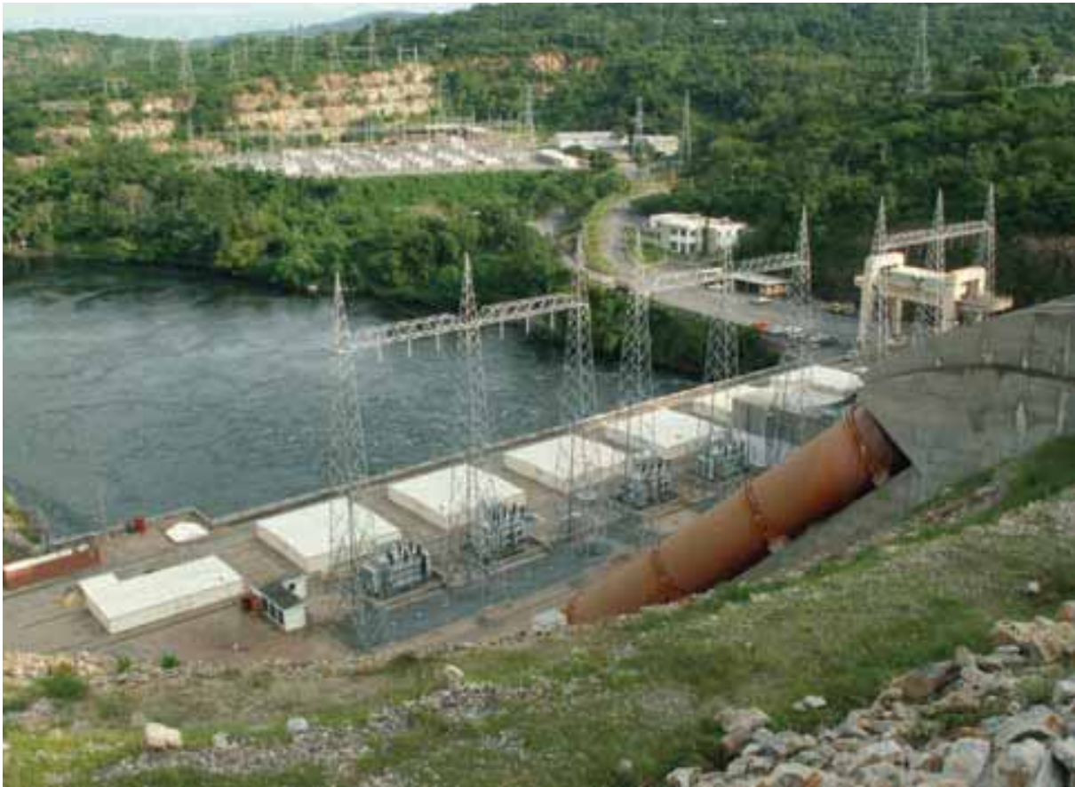
The Akosombo Dam, on the Volta River, Ghana. The construction of dams has been identified as a major part of Africa's future development, however if this development is to be sustainable their impacts on ecosystems and biodiversity cannot be neglected. © KEVIN SMITH
