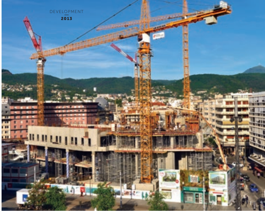
Extension works at the Jaude Center, in the very heart of Clermont-Ferrand.
