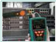
PoE switches & wire tracing
