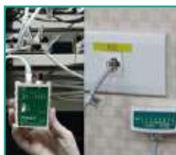
RJ45 cable test
