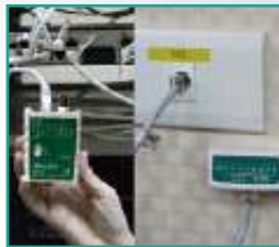
RJ45 cable test
