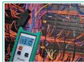
Fiber optic power test
