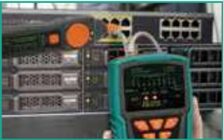
PoE switches & wire tracing
