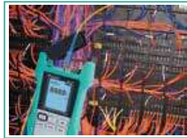
Fiber optic power test
