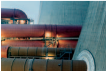
Purified gas lines leading to cooling towers
