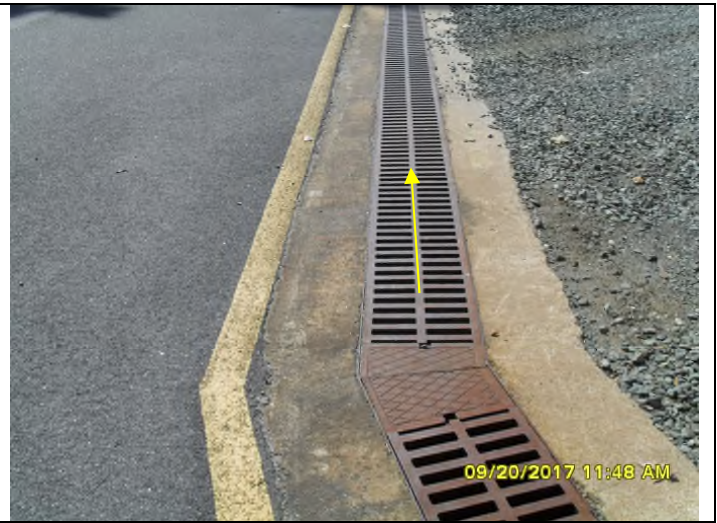
Photo 2. Trench drain from Internal Outfall 104 to retention pond. Flow is in the direction of the arrow.
