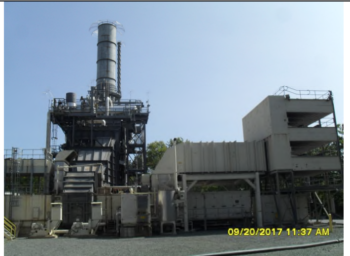
Photo 4. Unit 2. Boiler blowdown from this unit discharges to Internal Outfall 101.
