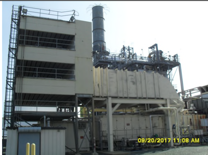
Photo 3. Unit 1. Boiler blowdown from this unit discharges to Internal Outfall 101.
