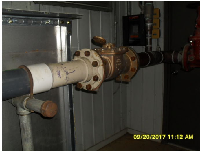
Photo 3. Town of Gordonsville water connection.
