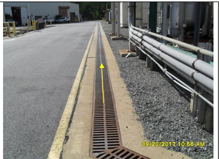
Photo 2. Trench drain from Internal Outfall 103 to retention pond. Flow is in the direction of the arrow.
