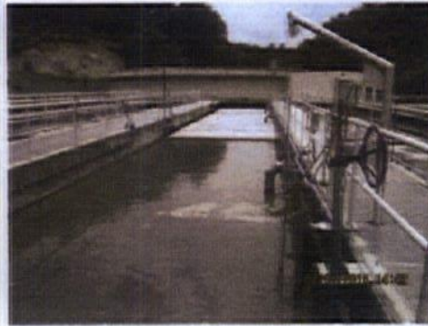
Activated Sludge Aeration
