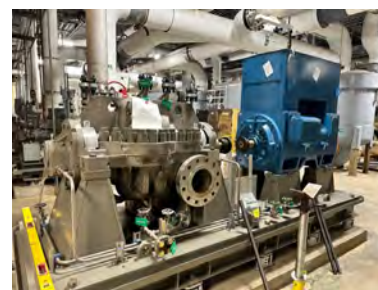
Figure 2.2.2.3. Magnet cooling water pump MCP1F and motor shown after being positioned and set on pad.
