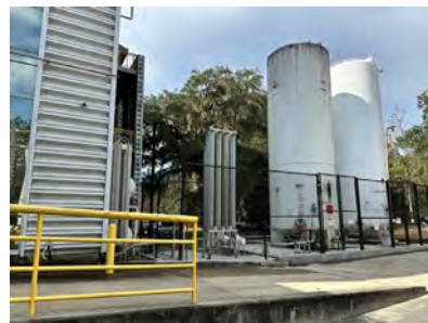
Figure 2.2.2.1. The new LN 2 tank (right-hand side) is shown installed alongside the existing LN 2 tank (left-hand side).
