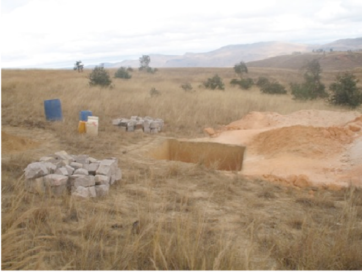
Figure 8 –First phase of the construction of the variometer vault, global view towards the South.
