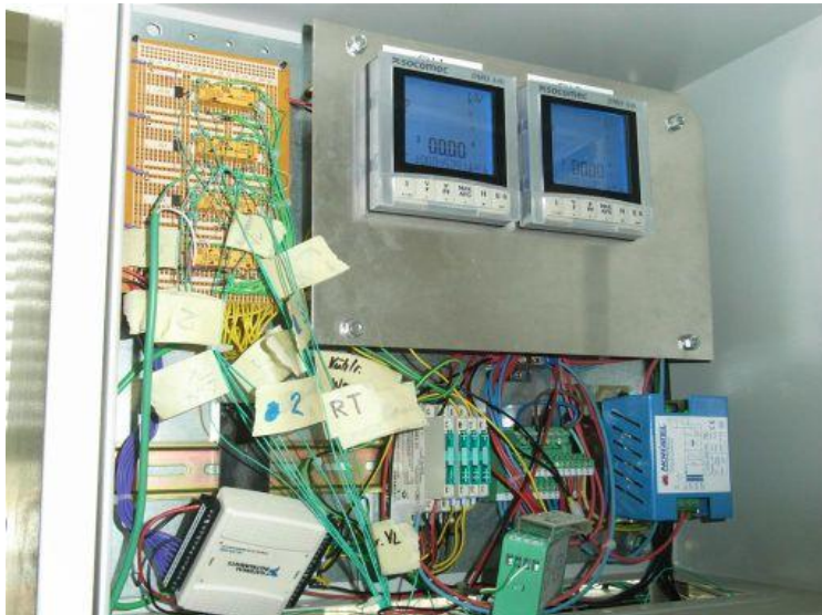
Fig. 5: Measurement and control system
