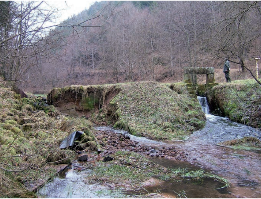
Fig. 9: Drift pond dam from the 19 th century with historical outlet structure (right side) and damage requiring restoration (left side).
