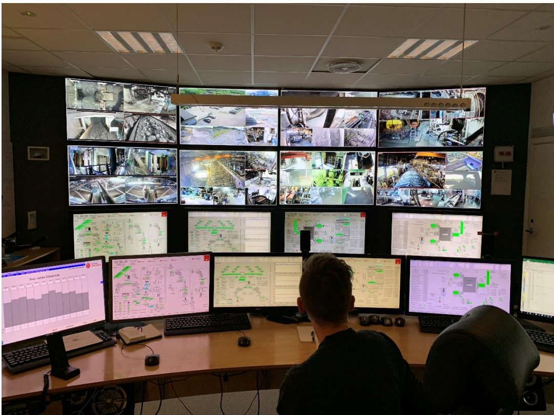
Figure 10-21: Process plant control room (Source: BGS)
