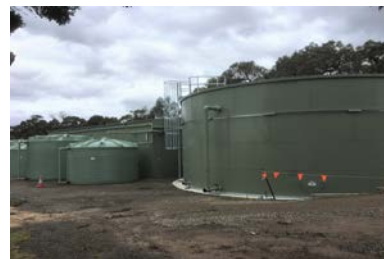
Water filtering plant, Cranbourne. Photo: Marjanne Rook
